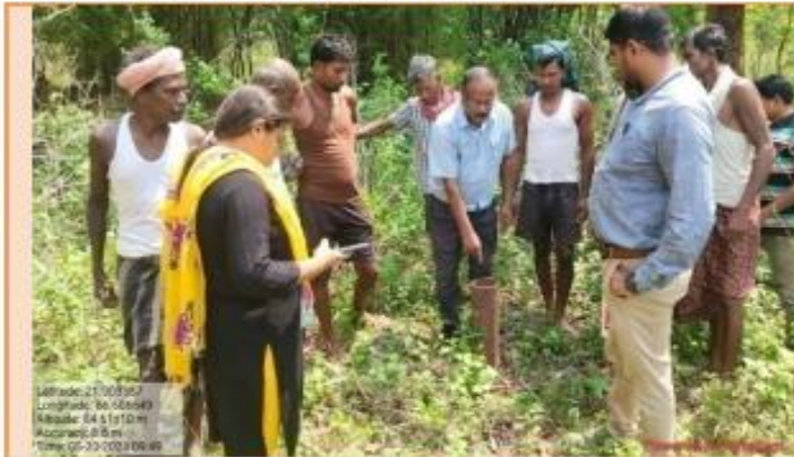
Solar Borewell site verification by Scheme Officer, Digdiga MIP under Shamakanta Block
